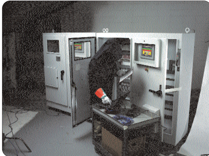
To deal with possible arc flash explosions, electrical engineers wear bulky, fire-retardant suit, gloves, face shield/goggles. This hot and uncomfortable gear makes service and maintenance time-consuming and cumbersome.
